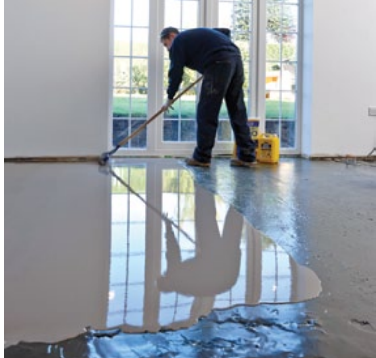
Floor prepared with STOPGAP F77 WSM, underlayment (STOPGAP 1200 PRO) being applied on top
