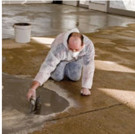
Applying a smoothing underlayment to a damp concrete floor prior to the application of a WSM
