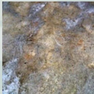
Laitance is a weak layer that may cause premature failure of a flooring installation
